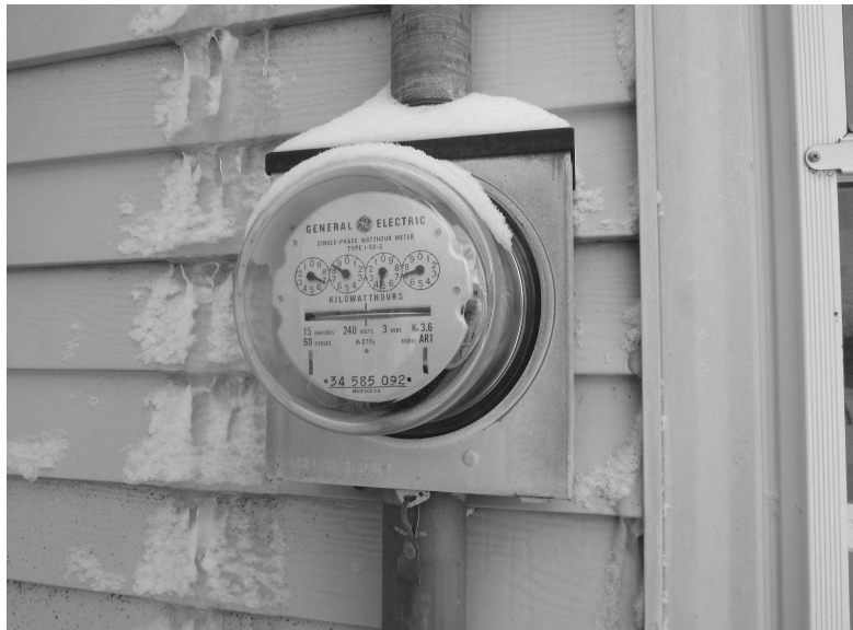
Meters like these will be upgraded in coming months to more efficient meters that will send messages electronically instead of requiring manual readings.
